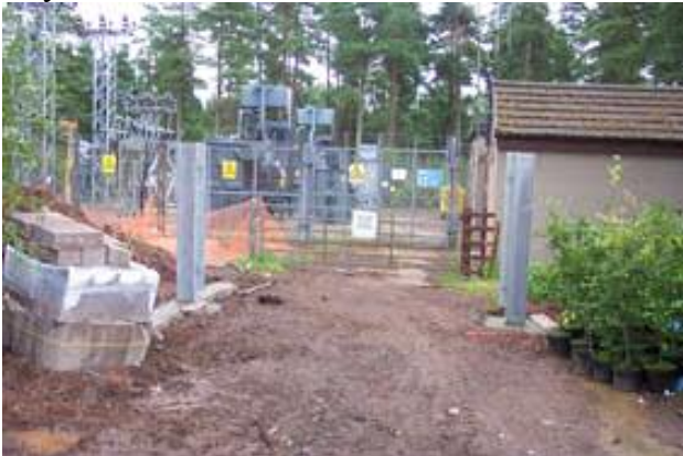
The noisy and unsightly substation is clearly visible prior to Green Barrier erection.
