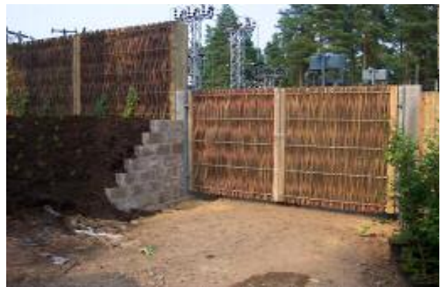
Sound attenuating gates incorporated, using the same high quality soundproofing material as the barrier.
