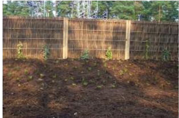
The 2m high Green Barrier erected on a 1.5m soil bund, softening the appearance and providing additional height to the acoustic screen.
