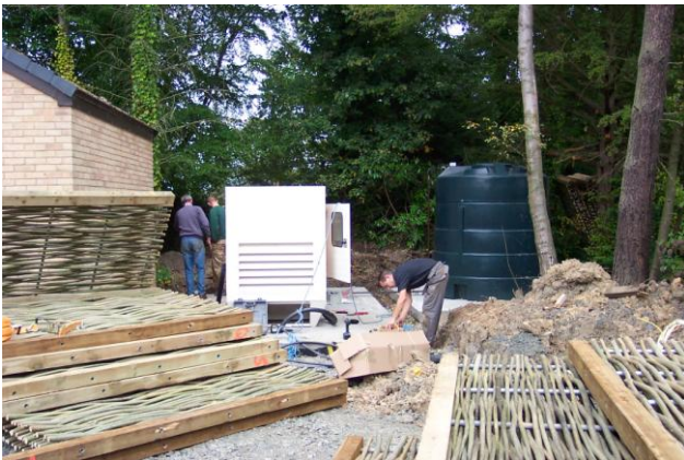
The large generator and fuel tank prior to screening.
