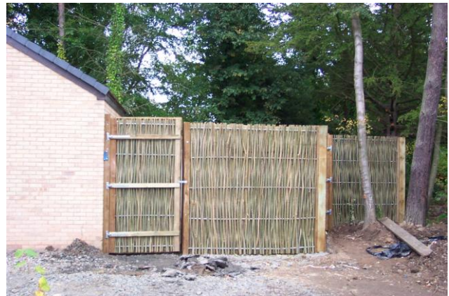
The acoustic protection installed together with an acoustic gate.
