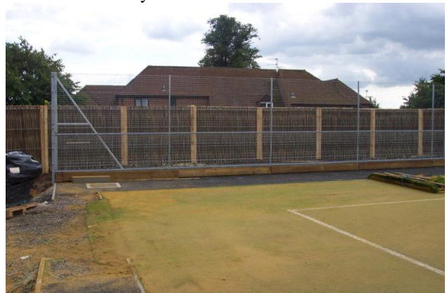
The Green Barrier™ reduces noise levels considerably for the residents of the nearby housing, and blends in well with the surroundings.
