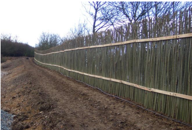
The 2.5m height provides security and once covered in foliage will create an extremely dense hedge.
