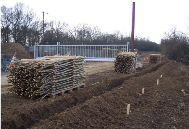
The trench prepared with the Willow panels laid out ready for erection.
